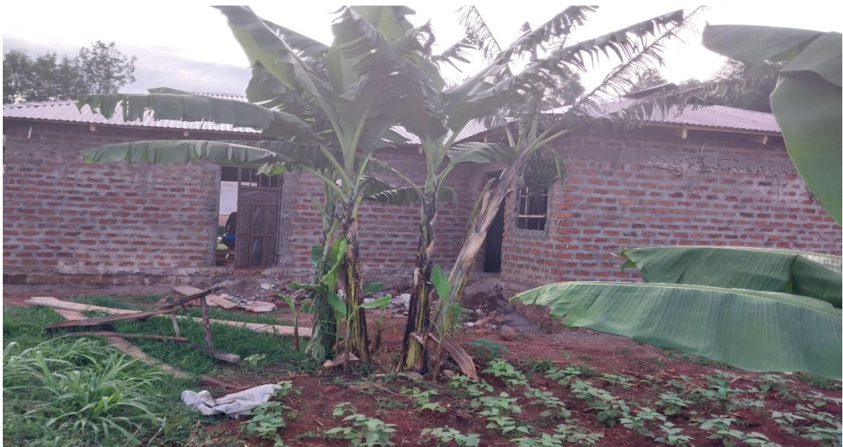
Rear view of the kitchen showing the cooks room. The kitchen roofed , door and windows fitted
